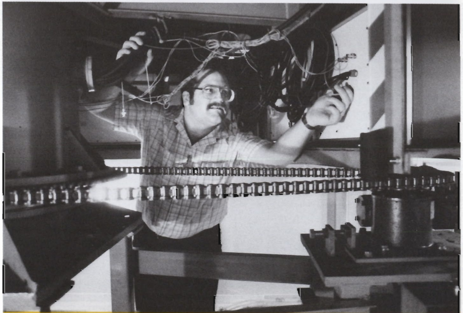
John Reynolds climbs down into the equipment pit under the 12-foot turntable to make electrical connections for the products which will be tested.
